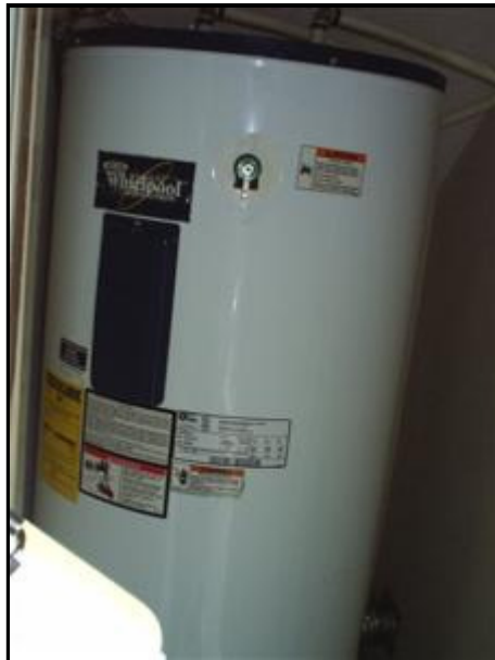
6.2 Picture 1 Water heater located in garage
