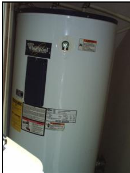
6.2 Picture 1 Water heater located in garage
