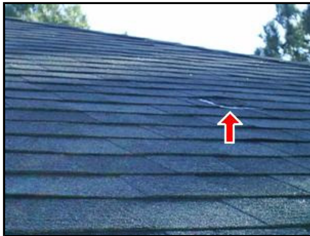
1.0 Picture 1 Deteriorating asphalt shingle
