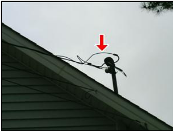
7.0 Picture 1 Electrical service entrance.
