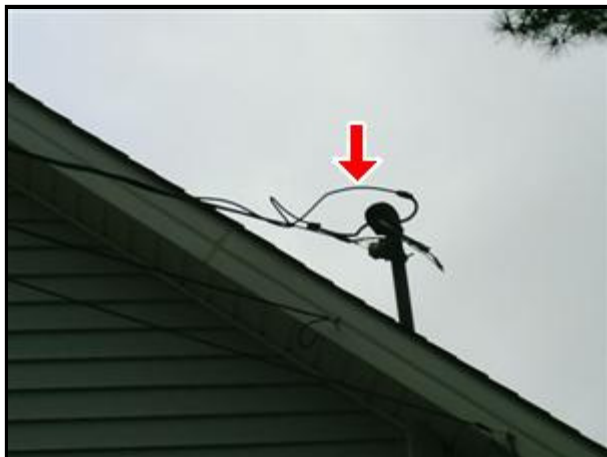
7.0 Picture 1 Electrical service entrance.
