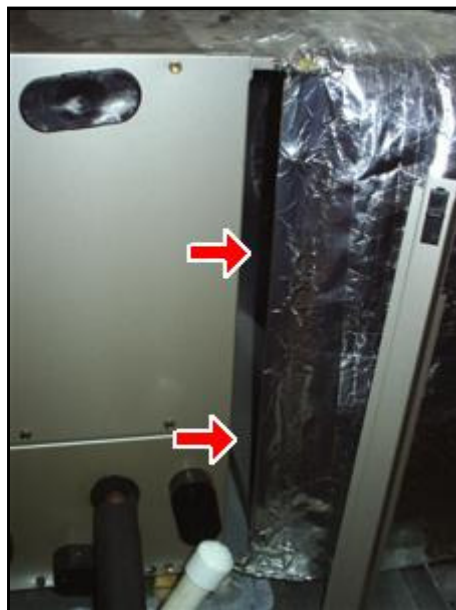
8.0 Picture 1 Heat pump attic
