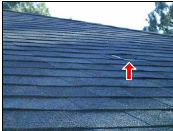
1.0 Picture 1 Deteriorating asphalt shingle
