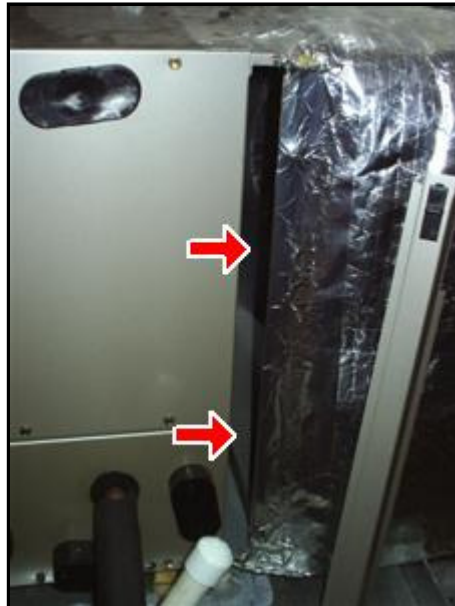
8.0 Picture 1 Heat pump attic
